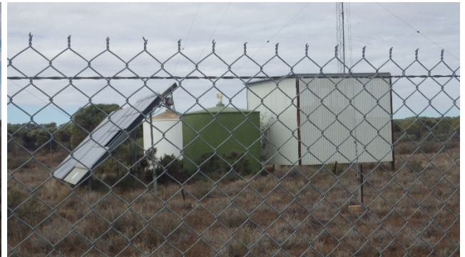
Photograph 16: RFDS radio towers - tanks and solar panels
